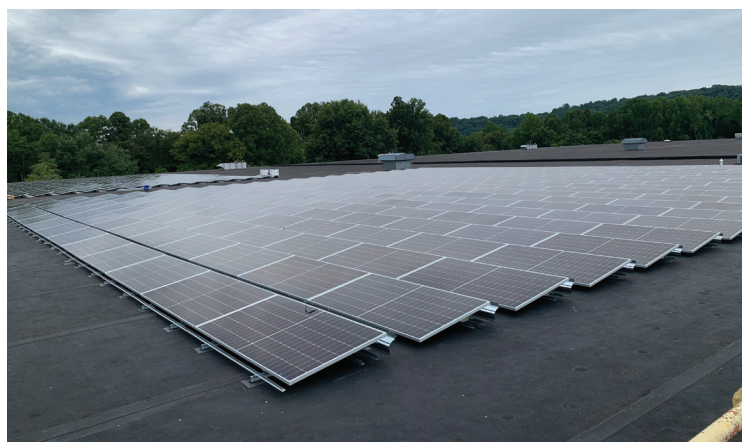
Davisville, West Virginia solar energy system.
